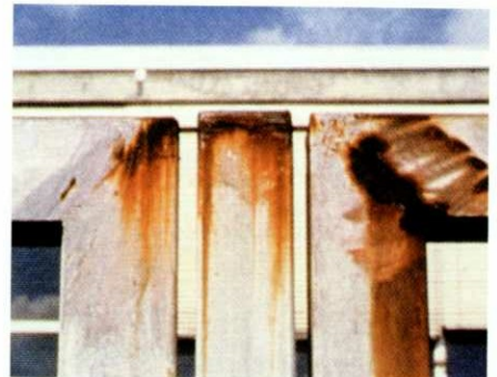
Fig 3: Where galvanized structures are welded, the steel exposed must be adequately protected (see text). Where this is not done, severe rust staining occurs as shown in this illustration.
