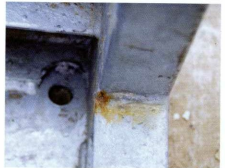
Fig 4: Seepage from pretreatment solutions from a weld
