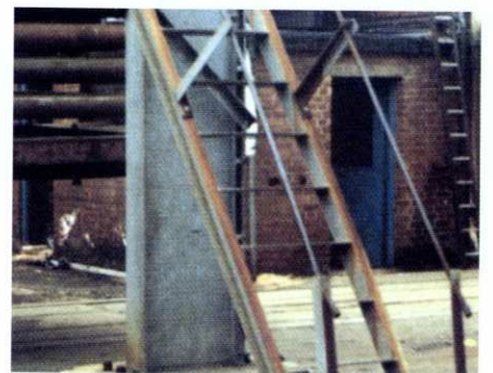
Fig 5: Water draining from rusting steel (out of picture) causes staining of sound galvanized surfaces of the stairway illustrated here.
